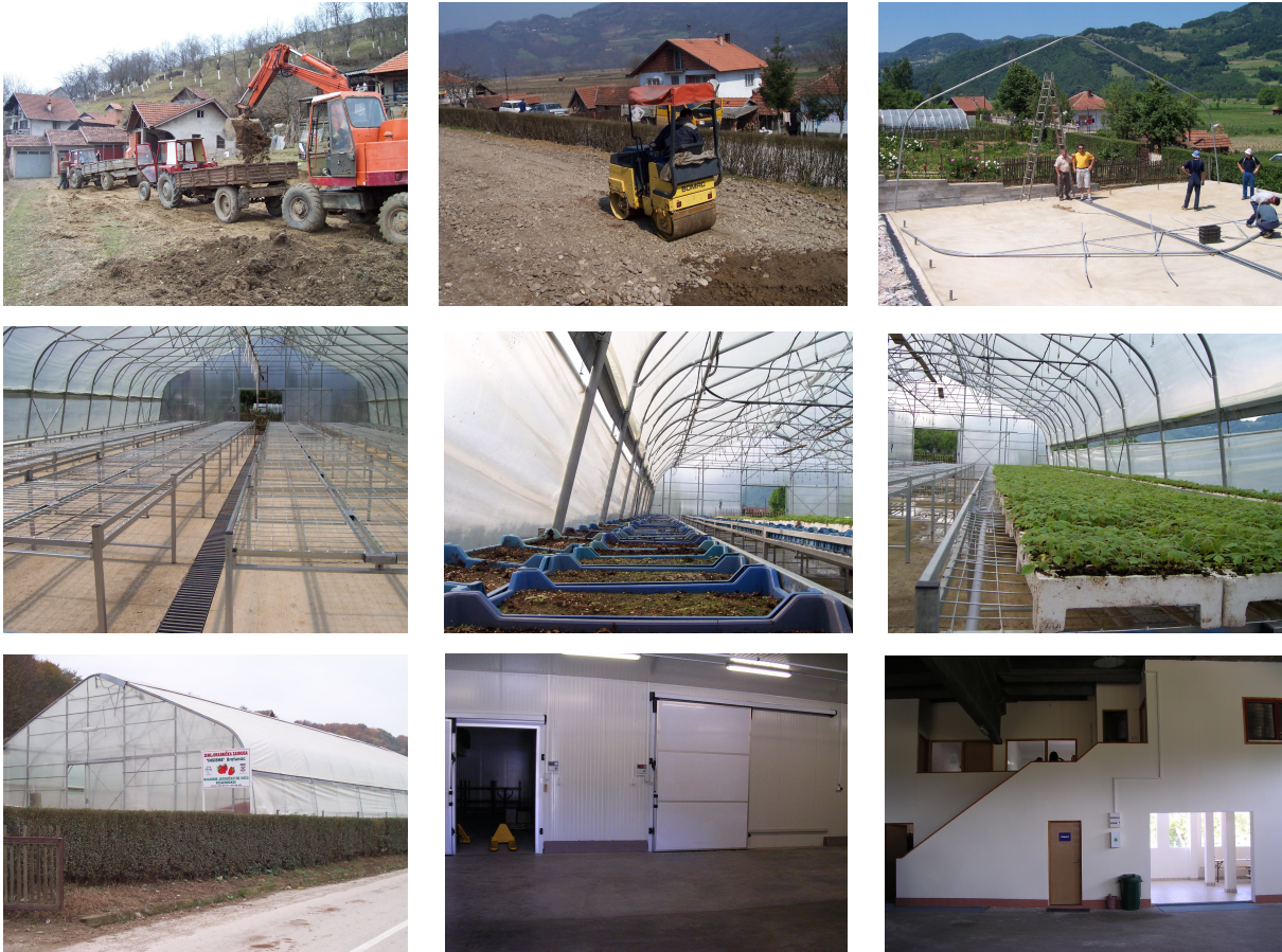
Four steps of the nursery construction; two pictures of the cultivation of raspberry trees inside the nursery; a view of the nursery; the refrigeration system; the offices
